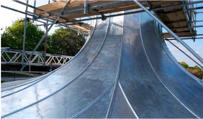
Figure 13 A zinc roof being added to a bandstand showing the colour of new zinc roofing.
