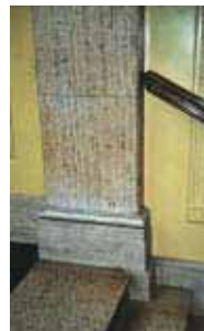
The original handrail at the Walker Art Gallery does not comply with current profile recommendations and does not project 300mm beyond the top riser because it abuts the pilaster. No changes have been proposed as a nearby lift provides alternative access.
