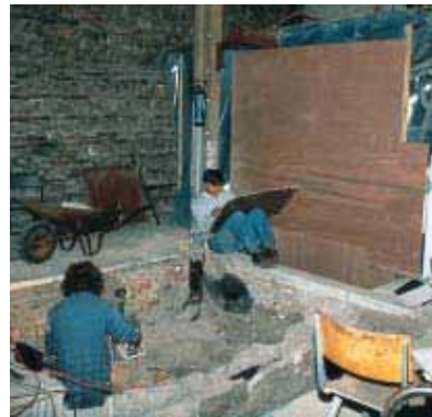
Consent for the insertion of a new passenger lift at Colchester Castle was dependent upon the outcome of an archaeological investigation. The cost and time to conduct an investigation needs to be anticipated in the building budget and programme.
