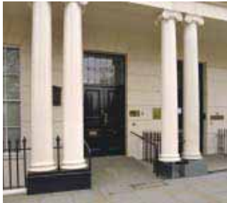
At the John Nash-designed Park Crescent near Regent's Park the space within the porch was deep enough to allow a short ramp over the single doorstep but insufficient to allow a level landing in front of the door. The handrails are utilitarian but they are integral with the ramp – a cheap but reversible solution.
