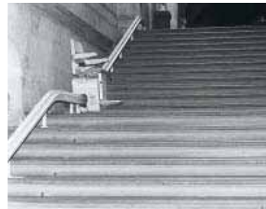
Incline stairlifts are inevitably intrusive and cannot be used by those unable to transfer from their own wheelchairs. However, the scale of the staircase here means that the lift is less intrusive than it might be elsewhere.
