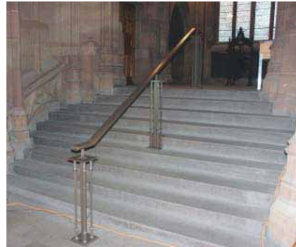
This photograph shows a mock-up of a proposed handrail for the staircase at the Grade I-listed John Rylands Library, Manchester. The handrail has been designed to relate to the very high-quality bronze work at the library and it is proposed that concealed lighting will be incorporated in the handrail to increase illumination of the stairs. Producing a mock-up provides a good way for all parties to assess the visual impact.
