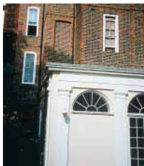
Substantial rebuilding at the rear of the Fan Museum in Greenwich provided the opportunity to add a rear lift shaft.
