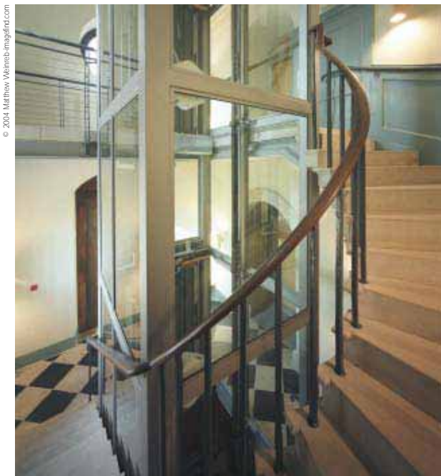
At St Luke's Church the rebuilding of an unsafe staircase allowed space for a lift, making all levels accessible.
