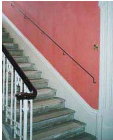
The addition of a second handrail improves access for ambulant disabled people on the historic staircase to the library at King's College Cambridge, though this does not fully comply with Approved Document Part M of the Building Regulations.
