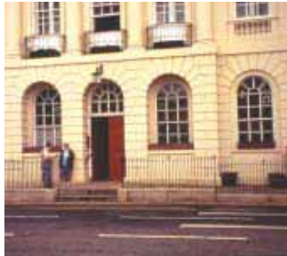
At Ripon Town Hall the whole pavement has been ramped up to threshold level over the original steps, part of an overall scheme that included the addition of a lift and accessible toilets inside. The increase in kerb height has necessitated railings but no handrail has been provided for the steps.
