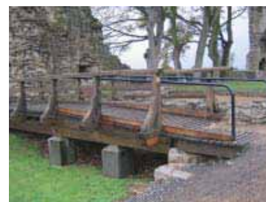
Barnard Castle. Modifications to the relatively modern bridge to the Inner Ward, which forms the main visitor route, replaced steps with a ramped solution. The use of circular section tubular steel handrails – although Approved Document Part M -compliant – is rather utilitarian.
