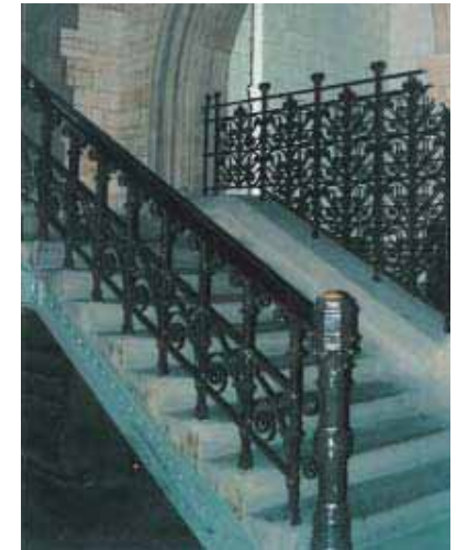
Manchester Town Hall. Although the original balustrade is to one side only and does not comply with standard guidance, the provision of a second handrail was deemed unnecessary because lift access is available within reasonable proximity to the primary circulation route.
