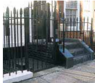
Many entrances to 18th-century and 19th-century terraced town houses have steps up to the front entrance, along with a basement area. An external platform lift was installed within the basement area of this London house, the steps and landing altered and the railings adapted in keeping with the existing design. A lift was installed within the house. The house has since been sold and the platform lift removed.
